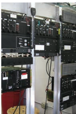
New Technology Radio System
