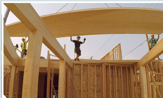
Mass timber construction in Bozeman, MT. Photo Credit: Brian Caldwell, ThinkTank Design Group
