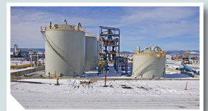
Red Rock Biofuel renewable jet fuel facility in construction. Photo Credit: Red Rock Biofuels
