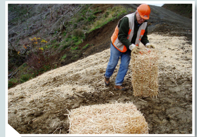
Wood straw product being hand applied for erosion control. Photo Credit: Colorado State Forest Service
